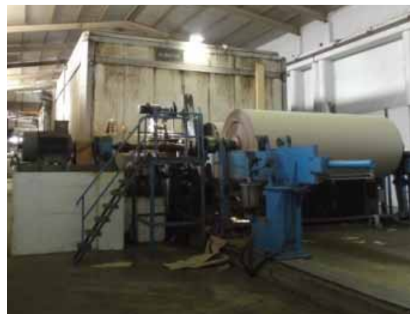
The continuous machine for texture paper production is the main steam consumer of the mill.
