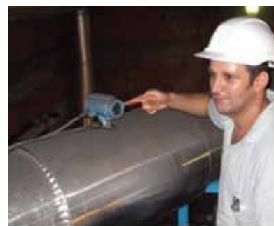
Rosemount 8800 MultiVariable™ Vortex installed in a saturated steam line coming from an auxiliary boiler.
