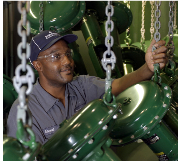
With full assemblies ready to replace the old valves in an instant, the turnaround was streamlined and the plant was able to get up and running on schedule.
