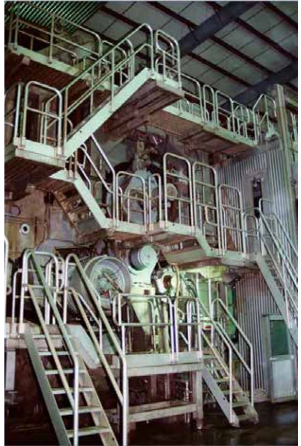
Pratt installed an OVER Meccanica four-drier type board machine at the Shreveport mill to produce high performance, lightweight linerboard from 100% recycled paper.
