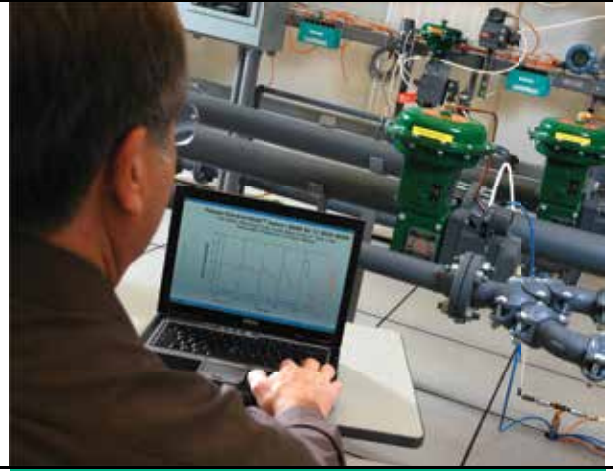
FIELDVUE™ digital valve controllers (background) provide Advanced Diagnostics to monitor control valve performance.
