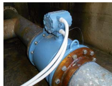
Rosemount Magnetic 10-inch flowmeter installed at Mediterranea delle Acque in the filtering area.
