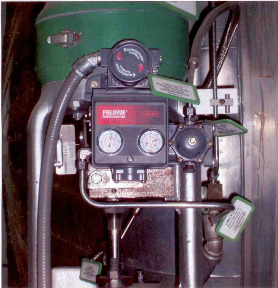
A globe-style reheater drain valve
