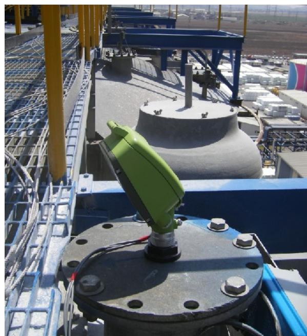
3D Solids Scanner mounted on the silo
