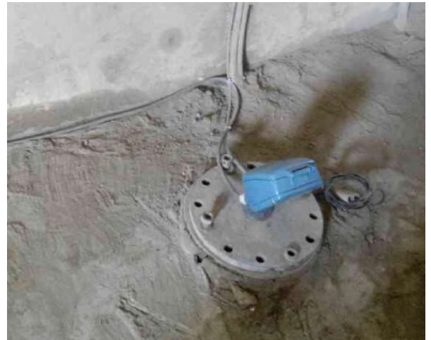
Rosemount 5708 installed on the cement silo
