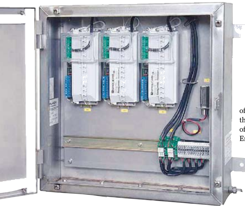
A BP floating production, storage, and offloading vessel will get FieldConnex fieldbus interface solutions from Pepperl+Fuchs and Emerson.
