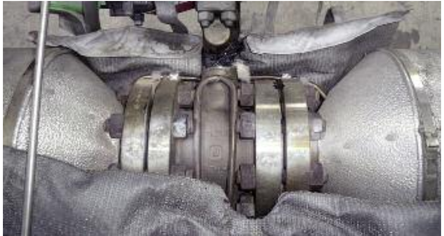
Figure 1. Removing insulation from around the ball valve in question revealed leakage locations.
