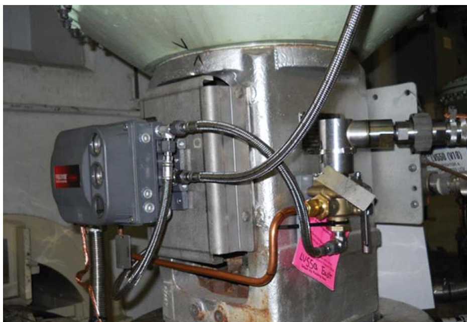
Figure 4. Since the digital valve controllers and high-capacity solenoids were installed, the Millstone plant has experienced no trips. The instruments provide data about valve performance and alert operators of any problems.
