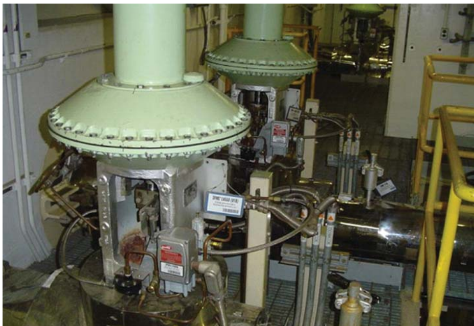
Figure 3. The original feedwater recirculation/startup valve assemblies at Millstone included problematic positioners, exhausts, and solenoids. The unreliable combination of instruments required manual control during startup and resulted in costly delays or plant trips.
