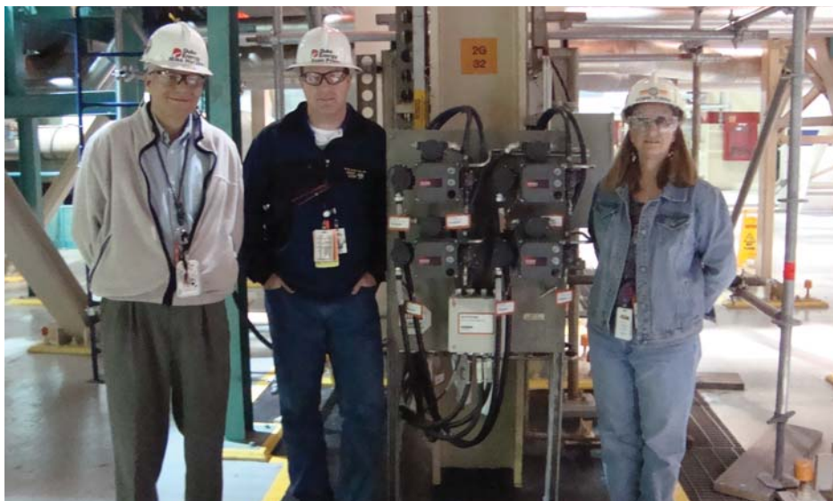
Figure 1. The dual redundant set-up and indicator station installed at the Duke Power site. Pictured are Mike Harazim (left), Robin Turpin, and Ryan Printy.
