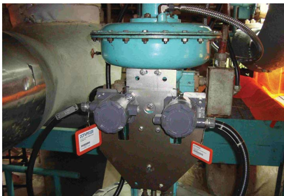
Figure 2. The dual redundant feedback sensors on the valve.
