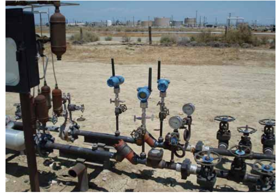
3051S WirelessHART pressure transmitters on a dual injection stream well.
