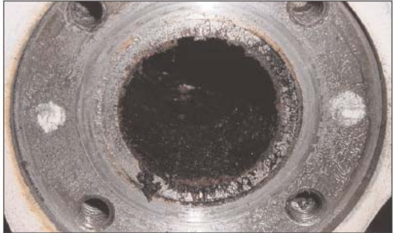
Upon inspection of the transducer ports, there was a very oily, gritty buildup of material.
