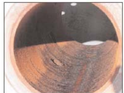
The photo above shows the buildup found on the meter.
