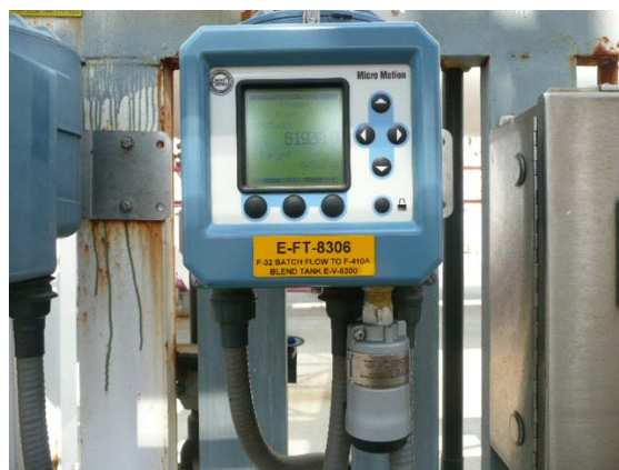
Micro Motion Model 3700 transmitter/controller installed with Smart Wireless THUM technology.
