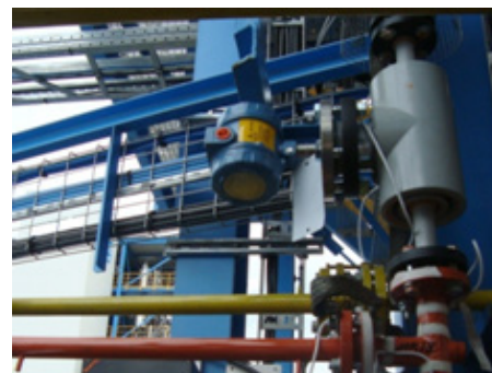
Zirconium Fork Density Meter Installation
