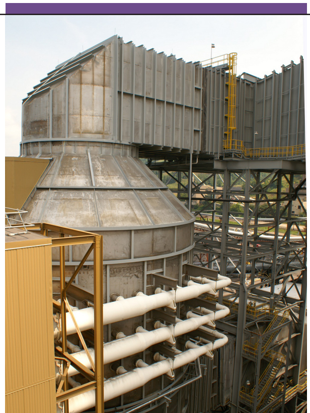
Absorber vessels, as shown above, were installed for both Mitchell units as part of the new FGD systems. The logic for this equipment was incorporated into the plant’s Ovation control system as part of the upgrade project.
