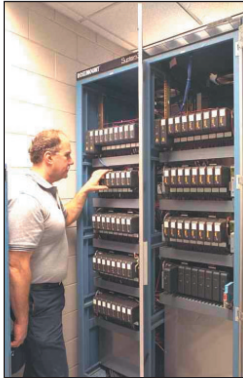
Figure 7. Cabinet containing two DeltaV™ controllers from Emerson Process Management, Systems Division, Austin, Texas.
