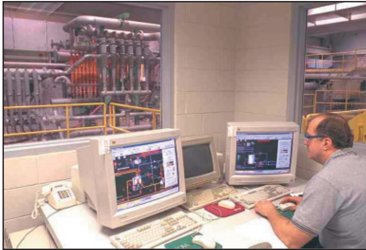
Figure 5. DeltaV operator stations in the pilot plant control room.
