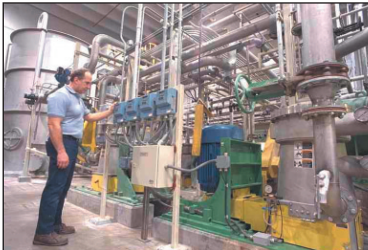
Figure 6. A shaft vibration/bearing temperature/kW/power factor analysis system instruments the pilot plant's newest Multi-Fractor screen and drive motor.
