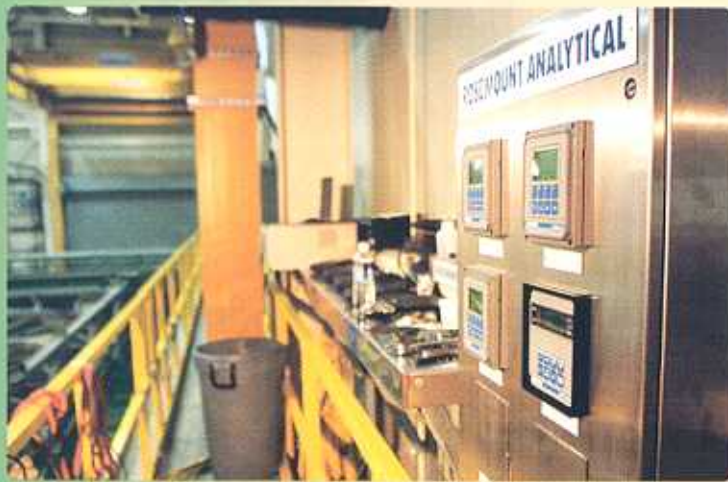
Rosemount Analytical devices being used to monitor the conductivity, pH/ORP and dissolved oxygen levels throughout the critical chloride removal.
