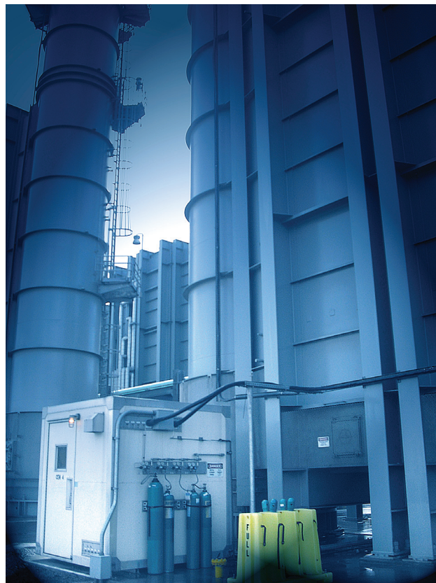
Figure 1. Continuous emissions monitoring systems (CEMS) must pass a certification test as part of the EPA certification process
