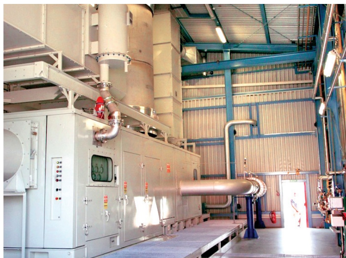
Enclosed Gas Compressor Building
