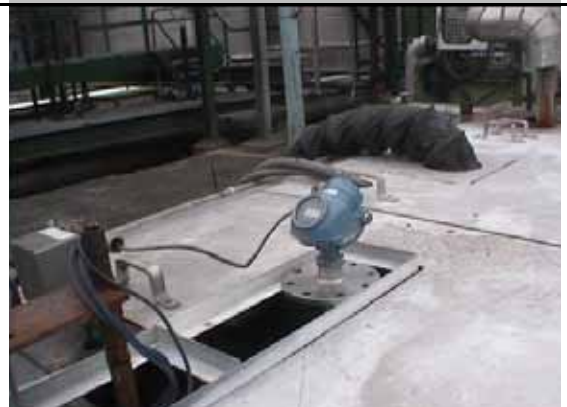
The Rosemount 5401 is installed over a wastewater collection tank.
