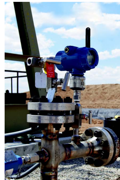
The Rosemount 3051S Wireless Pressure Transmitter Installed
