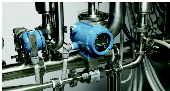
The Rosemount 8721 Hygienic Magmeter Installed.
