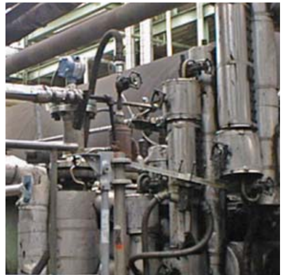
When first installed, the 3300 was mounted next to the displacer so both devices detected the same interface.
