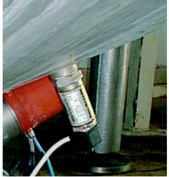
Signal is fed directly to the PLC via its PNP output.
