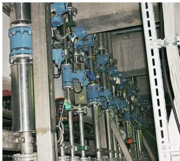
Rosemount 8700 Magnetic flowmeter systems installed at Stora Enso.
