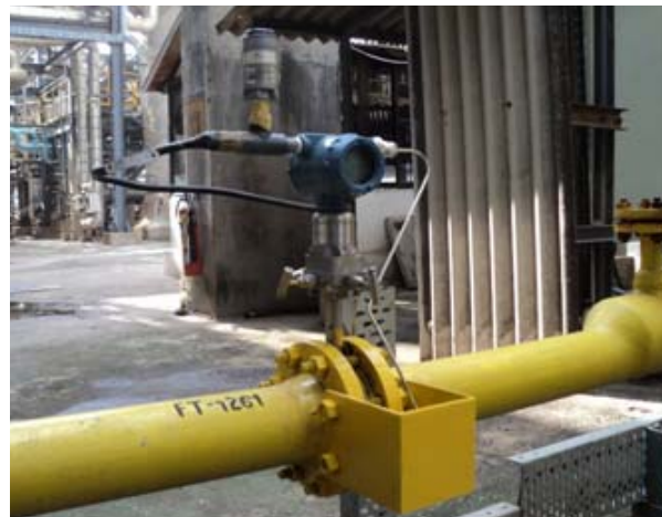
Wireless gas flow measurement with Rosemount 3051SFC and THUM was easily integrated into the plant DCS.
