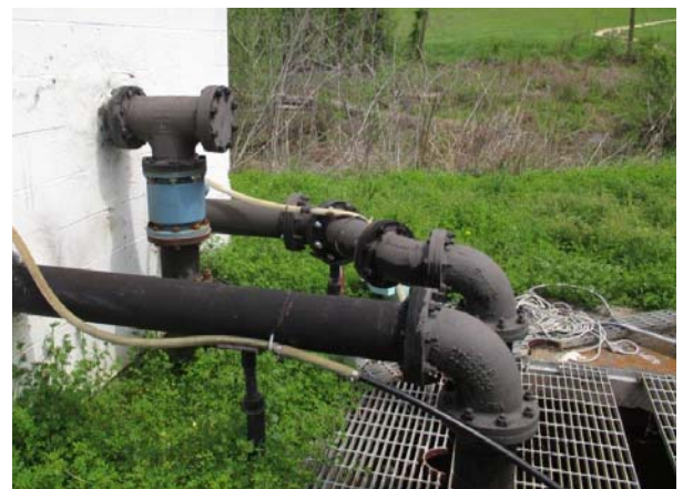
Flow meter installed in the discharge line leaving the station
