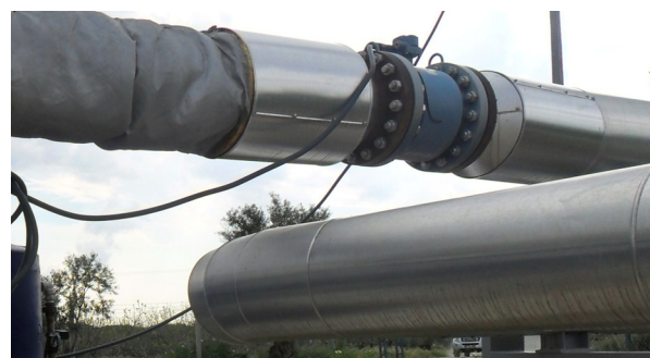
Rosemount 8705 Magnetic Flowmeter installed in the brine line
