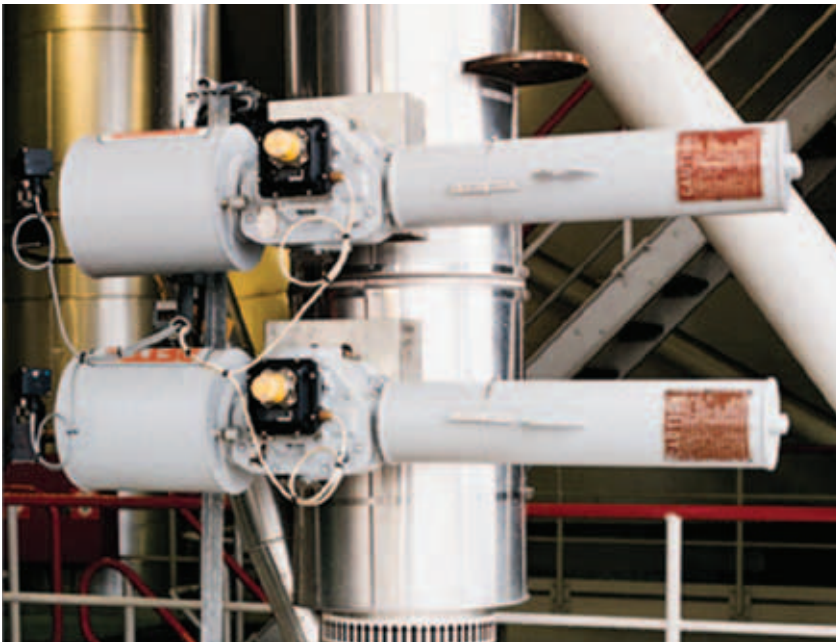
Redundant stem line pneumatic actuators.
