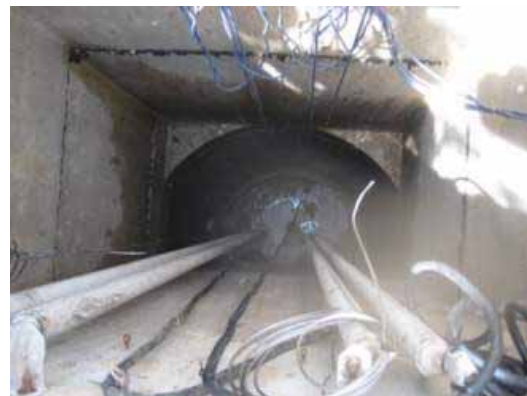
30-ft sewage lift station
