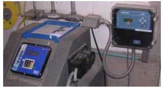
Figure 2. Rosemount 3491 controller used to calculate volumetric flow in the sewage line.
