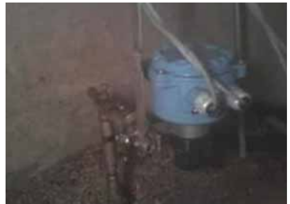
Figure 1. Rosemount 3102 installed on mill's sewer water line.
