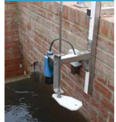
3108 High accuracy flow over weir
