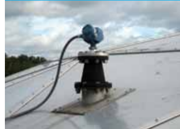
5400 Sludge holding tank
