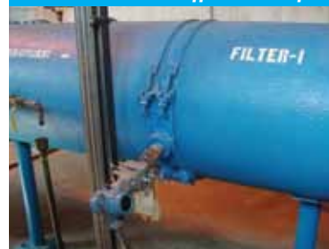
485 Annubar air flow to aeration
