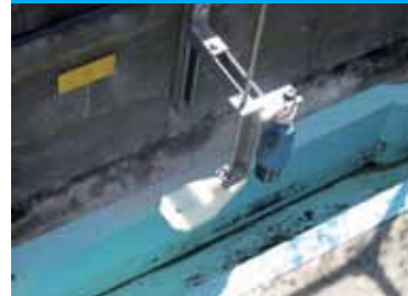
3107 Open channel flow
