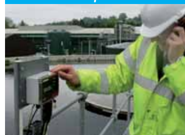
433S Sludge interface level
