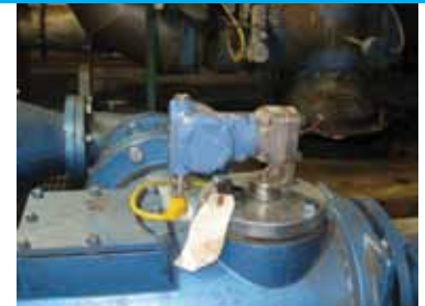
2051 Sludge pump pressure
