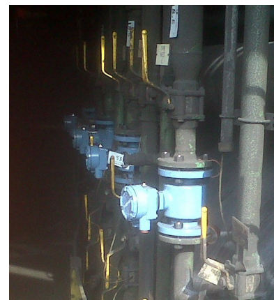
Installed Rosemount 8700 Magnetic Flowmeters at ArcelorMittal.
