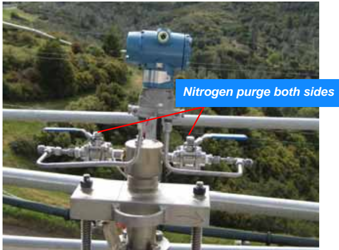
Figure 4. Nitrogen purges on high and low sides of the transmitter.
