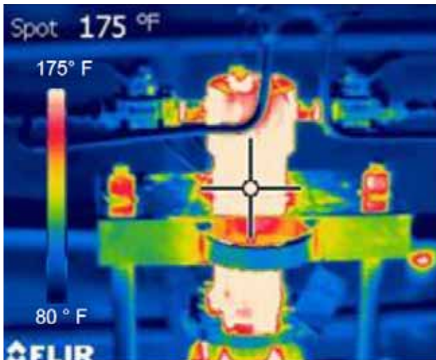
Figure 5. Thermal image photograph of the transmitter mounted on top of the pipe. The transmitter is well within its sensor limits of 250 °F. The temperature indication bar on the left of the thermal image depicts the range of temperatures present. Red indicates temperatures of approximately 110 °F, green indicates values of 100 °F, and dark blue indicates readings of about 80 °F.
