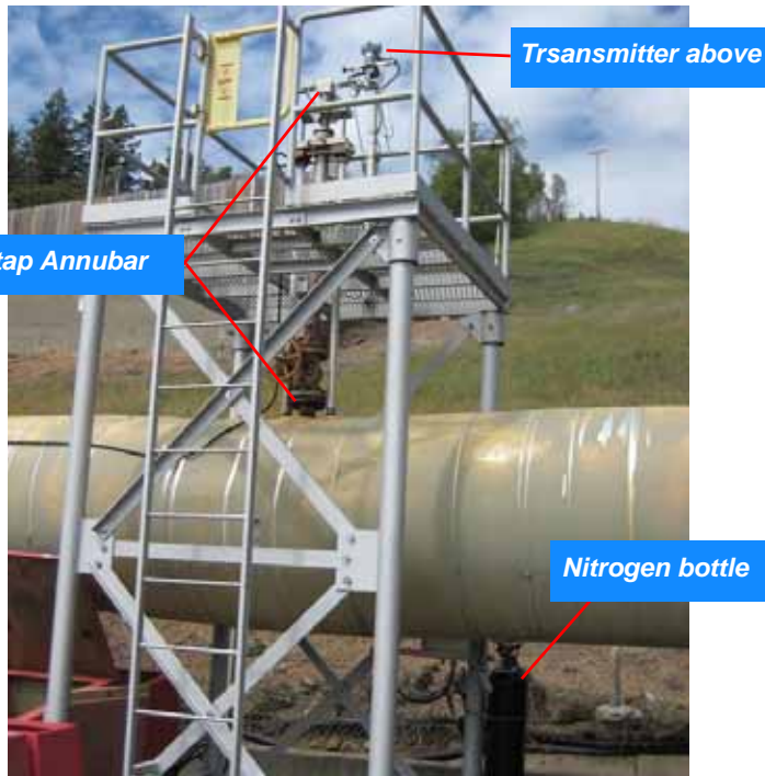
Figure 2. Close-coupled 3051SFA mounted in a geothermal steam application above the pipe. The process temperature in this application was 320 °F (160 °C). Figure 5 shows a thermal image picture of the same installation. This is well below the transmitter's sensor temperature limit of 250 °F (121 °C). This installation is for main steam turbine performance and has been in operation since January 2011 in the Geothermal fields in California.
