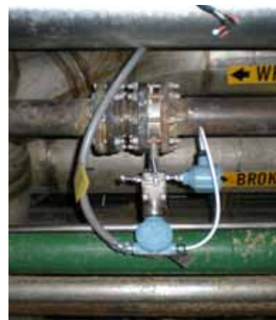
Figure 2: No new piping modifications or welding was required in this quick installation.
