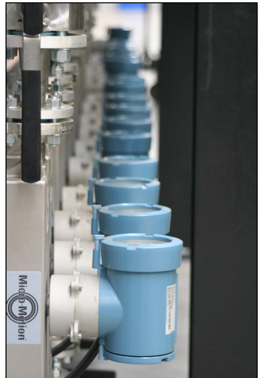
4/ A DETAIL OF THE DOSING SYSTEM WITH AN ARRAY OF MASS FLOW METERS
