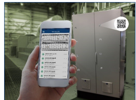
ATG View delivers asset health information to the user anywhere on the plant network.
