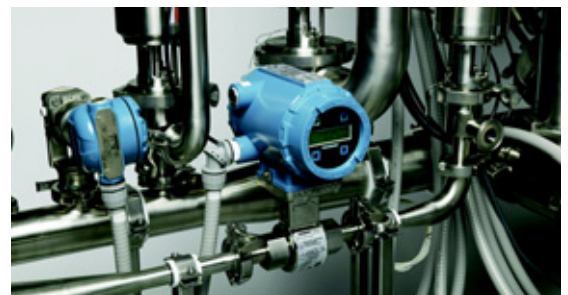
An installed 8721 Hygienic Flowmeter
