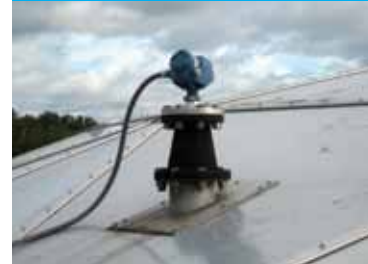
5400 Sludge holding tank
