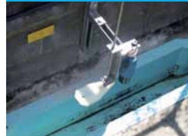
3107 Open channel flow
