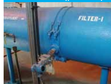
485 Annubar air flow to aeration
