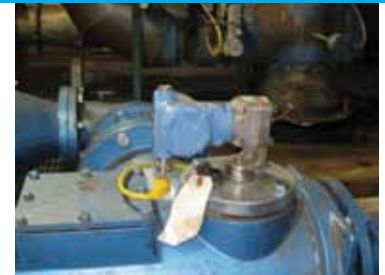
2051 Sludge pump pressure
