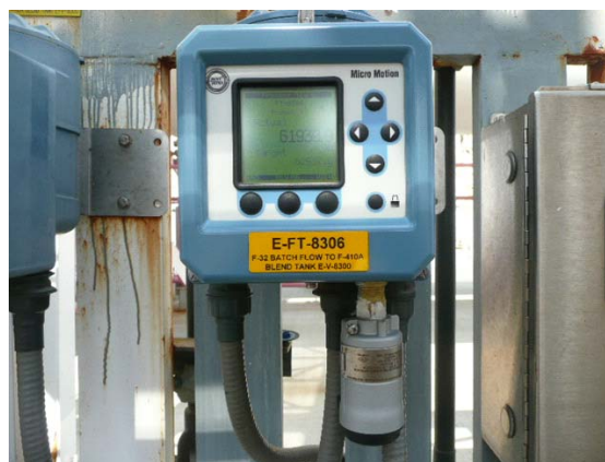
Micro Motion Model 3700 transmitter/controller installed with Smart Wireless THUM technology.
