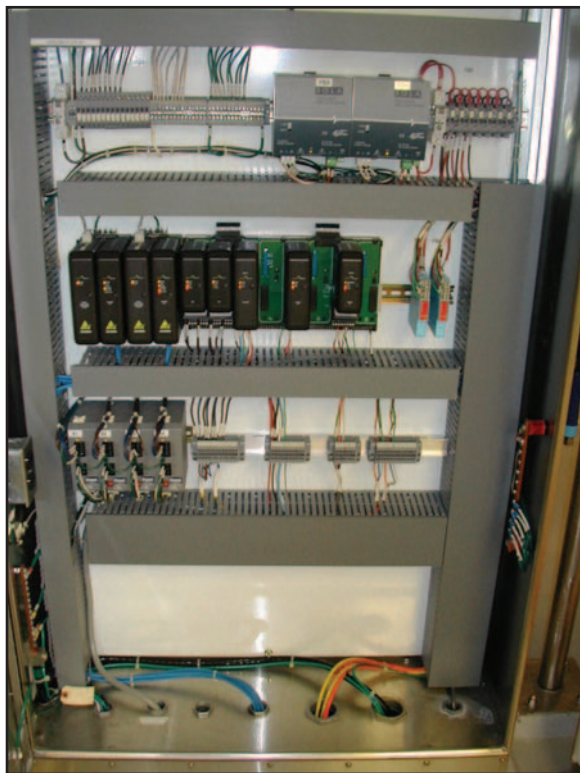
Fieldbus reduces the amount of space needed
