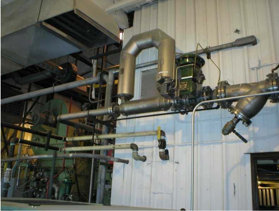
One of the 26 Micro Motion Coriolis meters with on-board Smart Meter Verification.
