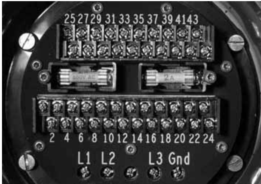
Figure 7-1 Fuses in the STC
