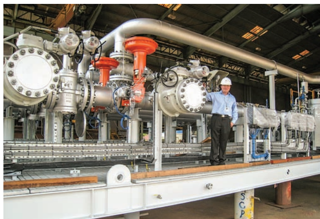
FIG. 5. This fiscal metering skid was assembled in a skid-building facility in Singapore and shipped to the refinery by boat. 1
