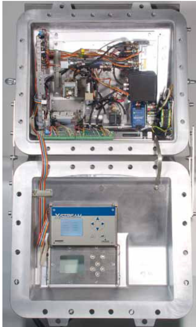
Interior view, showing 1 NDIR bench, 1 NDUV bench, 1 paramagnetic O 2 cell, thermostatic control (cover removed), analog and relay outputs, digital inputs, and serial interface.
