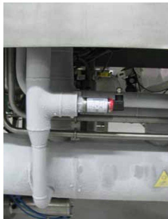
Figure 1. Installed Rosemount 2110 Compact Vibrating Fork Level Switch
