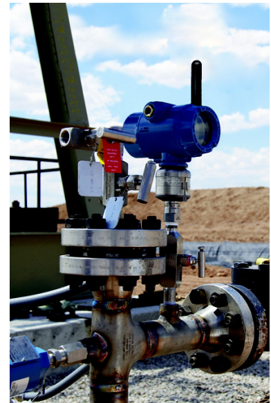
The Rosemount 3051S Wireless Pressure Transmitter Installed
