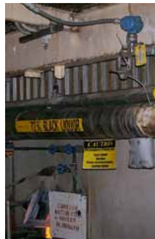
Figure 1. Installed Rosemount 1199 Gage Pressure Transmitter
