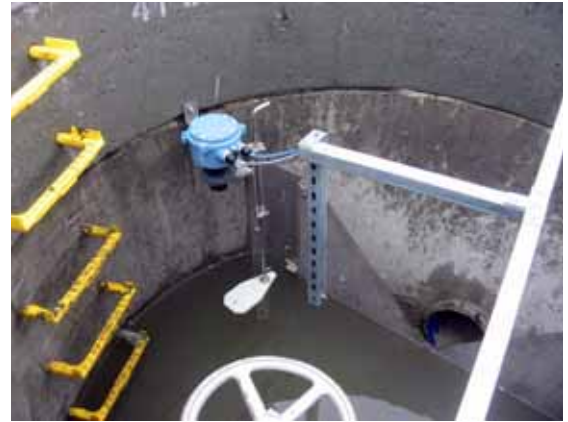
Figure 3. Final Installation with calibration plate and remote temperature sensor
