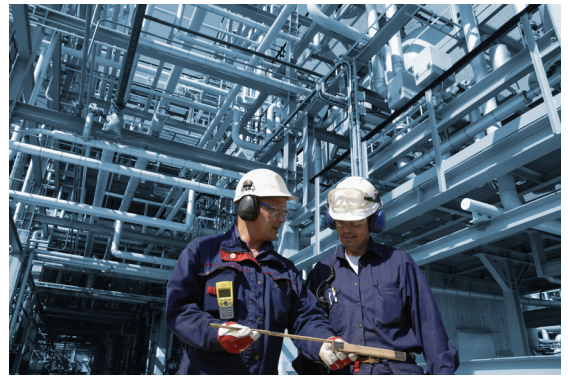
Dense piping, vessels, and tanks are a challenge to wiring, and to non-mesh wireless technologies
